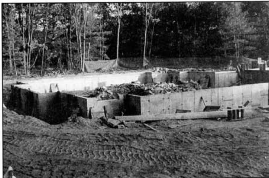
Meditation Hall site, late October, 2001. After compaction, footings and frost walls defined the shape of the Hall, sized to accommodate 65 yogis.
