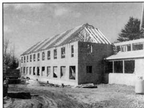
Retreatant accommodation, late Winter, 2002. Construction of the housing, located next to the Meditation Hall, continued through the cold months.
